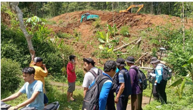
0-1. WILL BE RELEASED: Process of measuring land in Wadas Village for the construction of the Bener Dam project on Tuesday (11/4). In total there will be 124 hectares of land that will be used for the Bener Dam. (BPN Purworejo for Purworejo radar)
